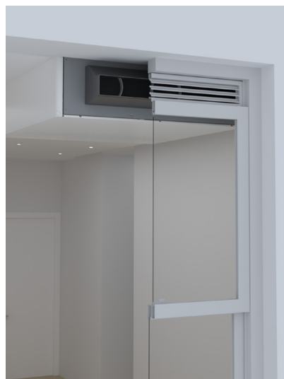
Direct existing window vent
